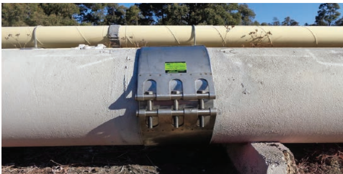
MJDL EPDM + strip insert 507mm. ash slurry line. 1km heavy weight fiberglass pipe of a coal fired power station. Australia
