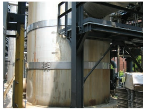
MJFL Viton 3,615mm. chemical storage tank. for protection of weld. Korea
