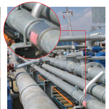
MJG EPDM 100A. sprinkler line for deck wash. Netherlands
