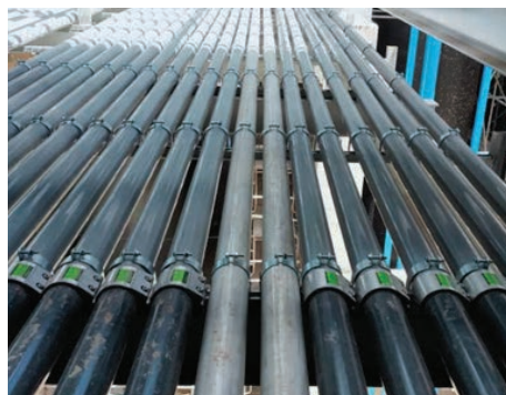
MJGL EPDM 50A, 80A, latex and coagulant conveying line, UPVC pipe, Malaysia
