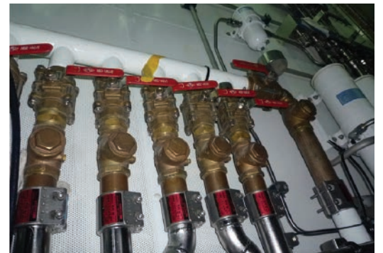
MJG NBR 40A. engine room. Taiwan
