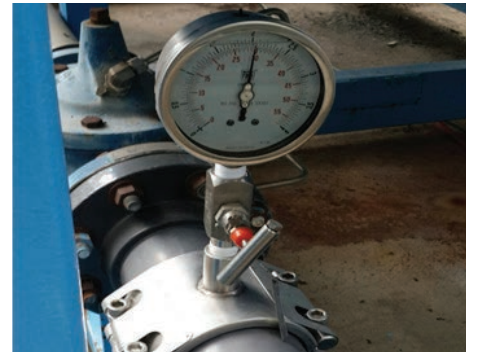
MJD-A EPDM 100mm. pressure gauge installed on PVC pipe. water supply line at power plant. Thailand
