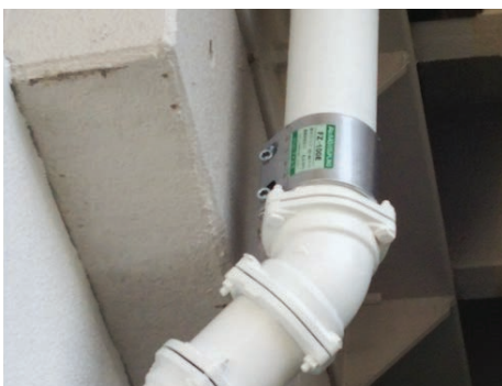
MGLP EPDM 100A, rainwater drainage pipe under overpass, Japan
