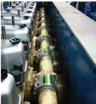
MJG EPDM 100A. engine room. Australia
