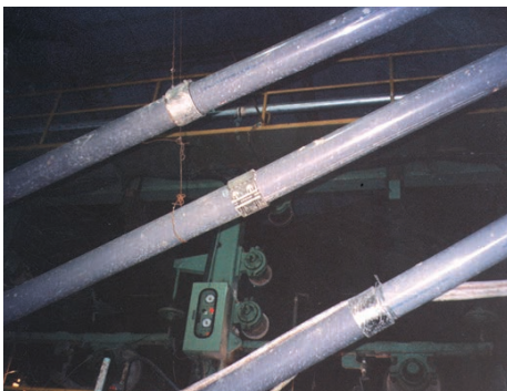
MJS EPDM 200A, pulp conveying line, PVC pipe, couplings used for pipe connection for pipes to be cleaned regularly, Korea
